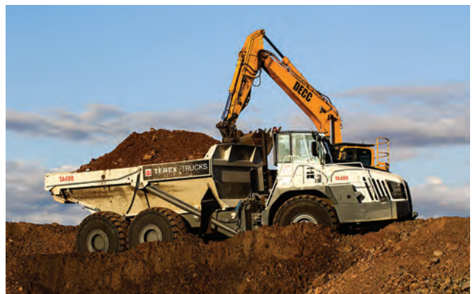
ALL IMAGES: The TA400 articulated hauler helps DECC to carry out a variety of jobs from remediation of landfills to stormwater management, at a site just outside Brisbane, Australia.
