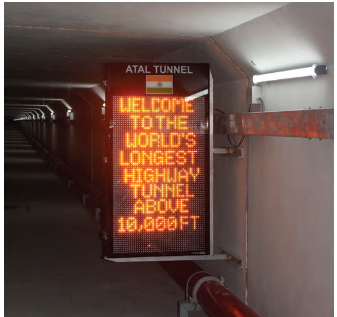
TOP AND ABOVE: The remoteness, accessibility and extreme altitude of the project presented immense challenges to geological works, tunnelling and mechanical and electrical installations.
