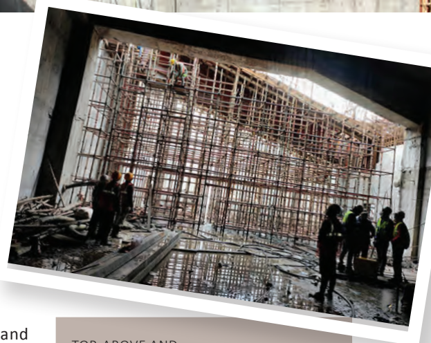
TOP, ABOVE AND BOTTOM LEFT: The drill & blast construction method was chosen for the project. Opened in October 2020, the tunnel now facilitates two-way traffic and can accommodate up to 3,000 vehicles per day in any weather conditions.
