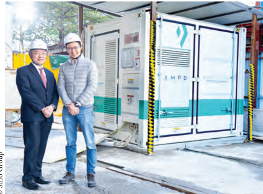
Andrew Young of Sino Group (on the left) and Brandon Ng of Ampd Energy visit the first of the Group's projects to adopt the Ertainer energy storage system.
