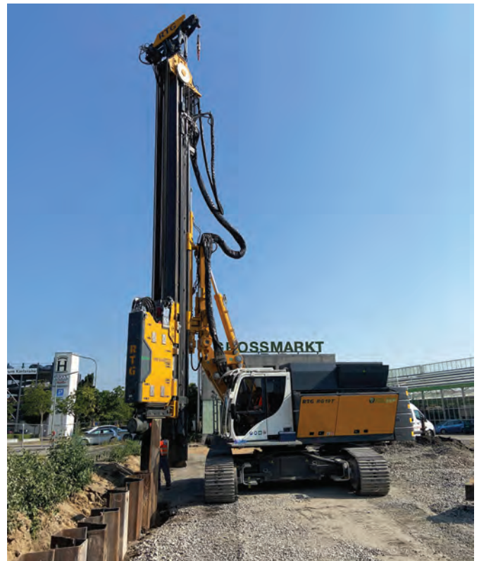
ABOVE: An RG 19T with the integrated sheet pile assistance system working on a project in Karlsruhe, Germany.
